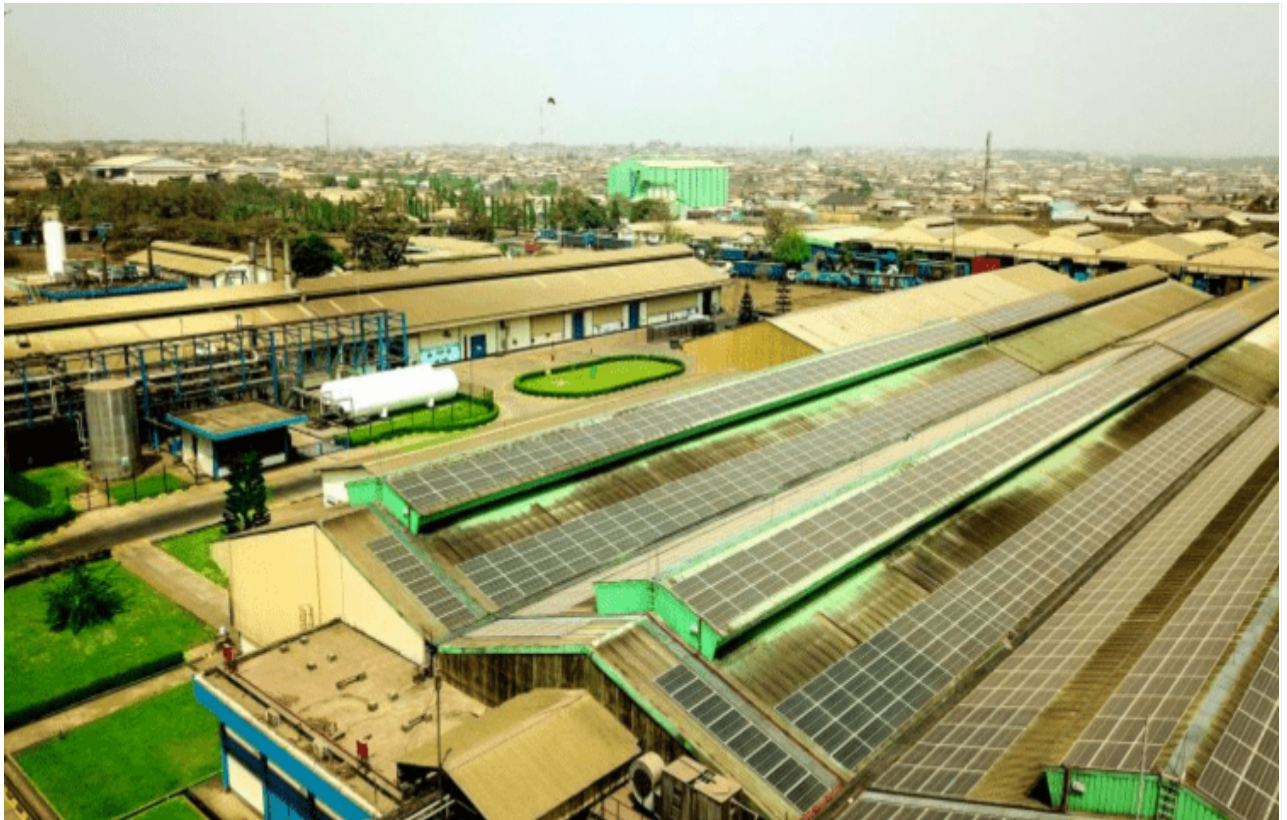
Nigerian Breweries Solar Power Plant, Ibadan
